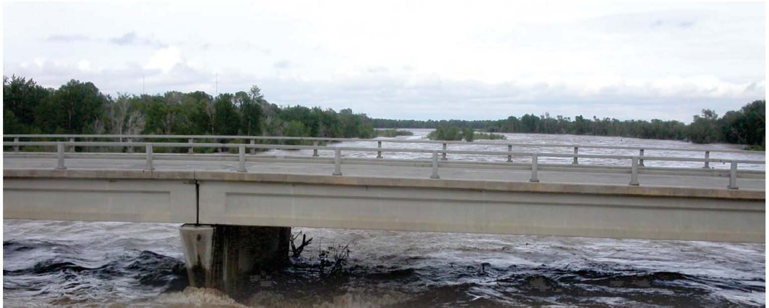
2005 flooding of Oldman River along Highway 2.
