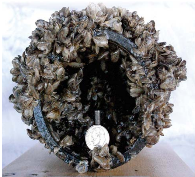
Pipe clogged with mussels.
