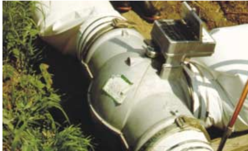
Surge valves can reduce erosion, improve the overall efficiency of surface irrigation and substantially reduce the amount of water needed for optimal yields.
