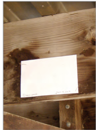
Figure 1.8 Example of a spot card placed on a beam in a livestock barn
