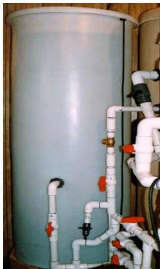
Figure 5 - Household Water Tank - 2 day water storage
