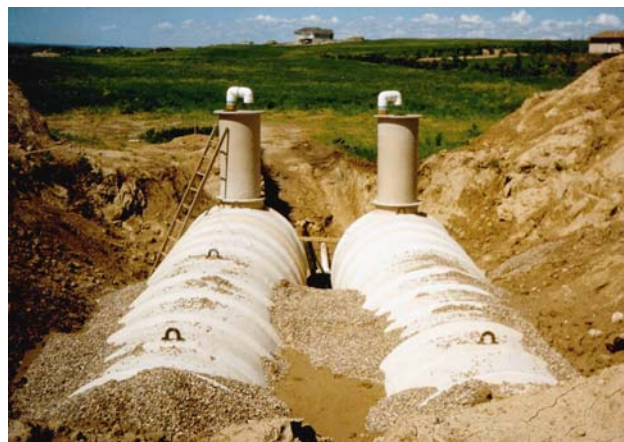
Figure 6 - Cisterns: Large volume water storage tanks
