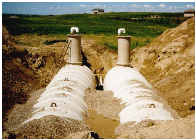
Figure 6 - Cisterns: Large volume water storage tanks
