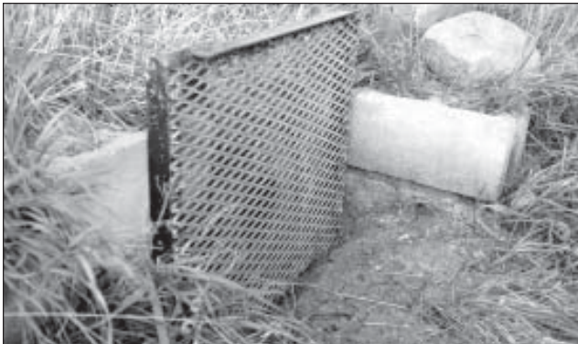
Figure 2. Farm ditch screen bolted to concrete structure
