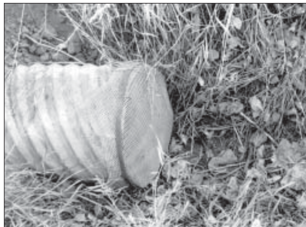
Figure 1. Culvert type screen installed on upstream end of culvert
