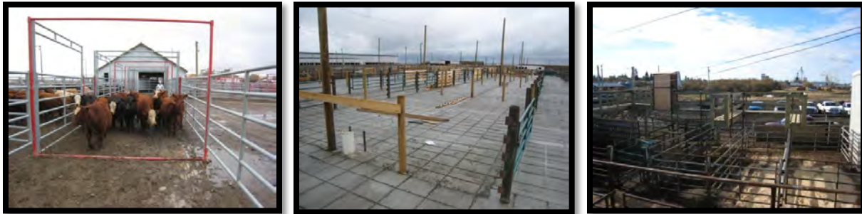
Picture 4, 5 and 6: Cattle leaving the scanning system to be penned (4), Construction of new pre-scanning pens (5), Scanning office built over the scanning pens (6)
