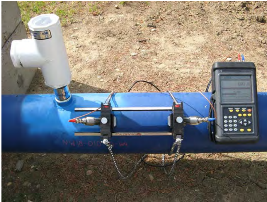
Turnout pipe supplying pivot in the SMRID with LOPAC flow monitor installed (right) and transit time flow meter measuring water flow (left).
