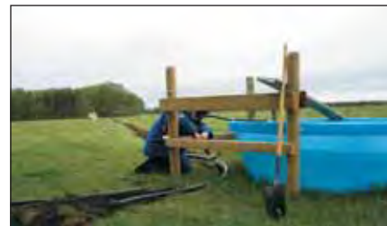
Water connection for trough
