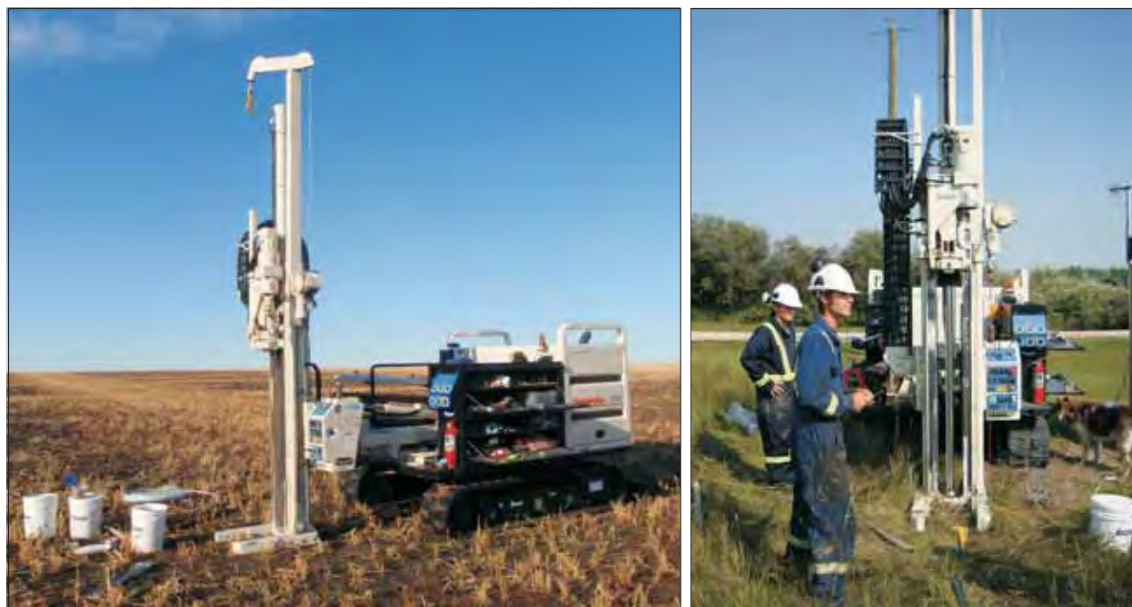
Groundwater wells were installed using a Geoprobe® 7730DT (a hydraulically powered soil probing unit), which allows installation with minimum soil disturbance.
